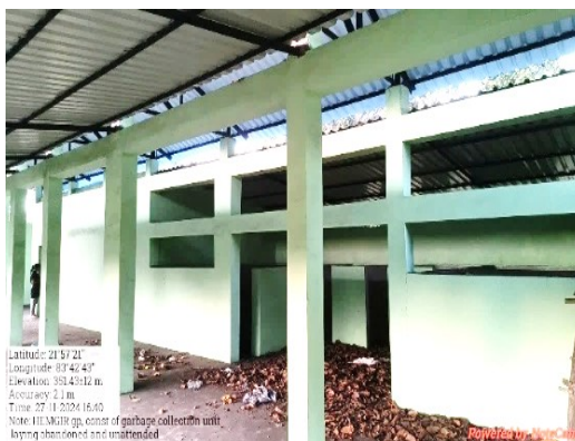
Picture 11: Abandoned Block level garbage collection unit at Hemgir Block
