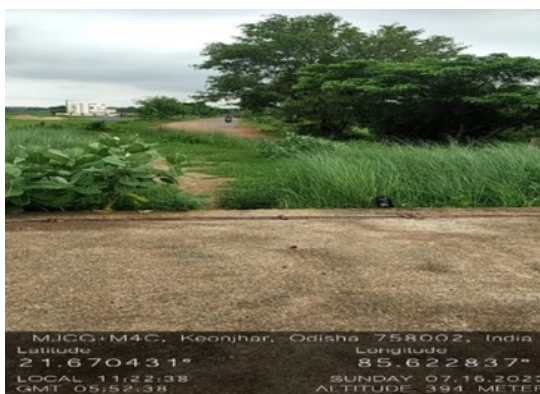
Photograph 8: Right side approach road not constructed due to non-acquisition of land
