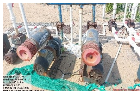
Picture 13: Non-functional STP at Chakratirtha beach
