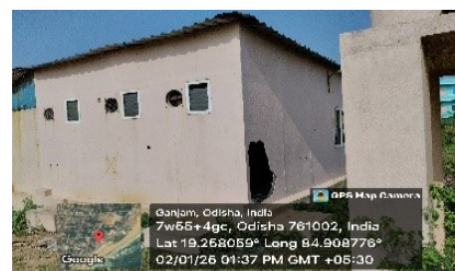
Picture 18: Non-functional of Police kiosk at Sea Beach, Gopalpur, Ganjam
