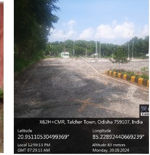
Picture-14: No direction sign at the testing track at Talcher
