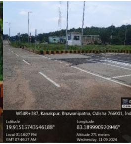
Picture-9: Damaged Testing track at Kalahandi (Bhawanipatna)
