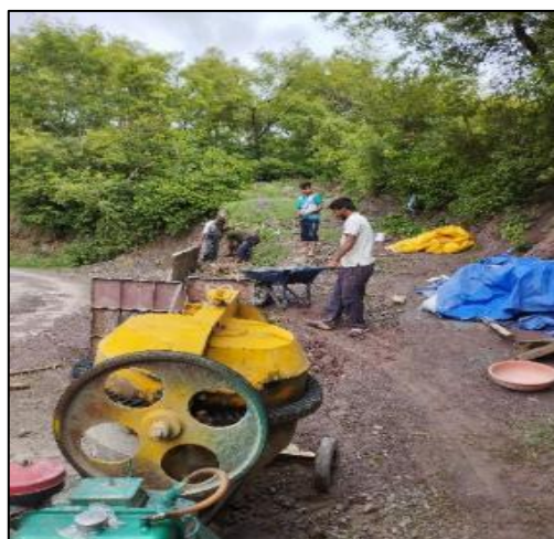
A picture uploaded on NMMS portal showing attendance of four workers while 10 workers were present in the e-MR No. 4516 on 10.08.2024 in GP Jadla (Solan)
