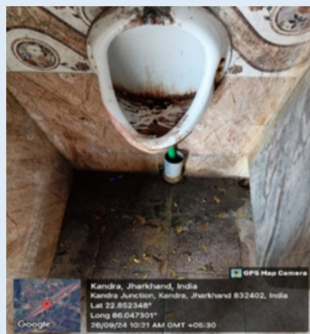
Fig. 3.9: Unhygienic urinal at Kandra (SER)
