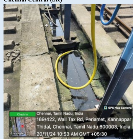
Fig. 3.7: Water hose lying in sewage drain at Chennai Central (SR)
