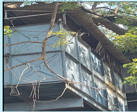
Fig. 3.13: Water tank at Palakkad (SR) not fully covered while trees adjacent to the tank were inhabited with bats and birds
