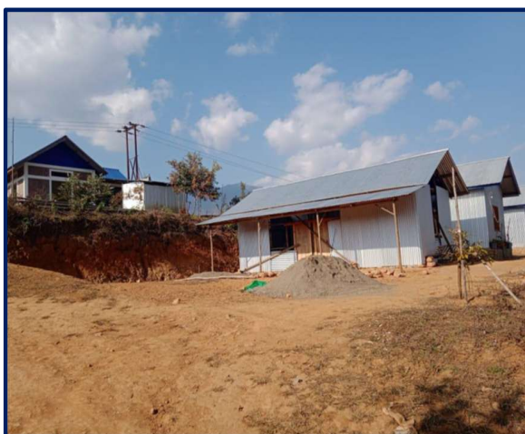
Picture 45 - Construction by encroachers
