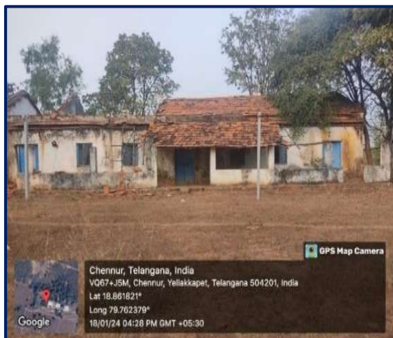
Coordinates - Lat – 18.861821°, Long – 79.762379° Picture 10 - Training Hall at BSMTC Chinnoor with collapsed roof
