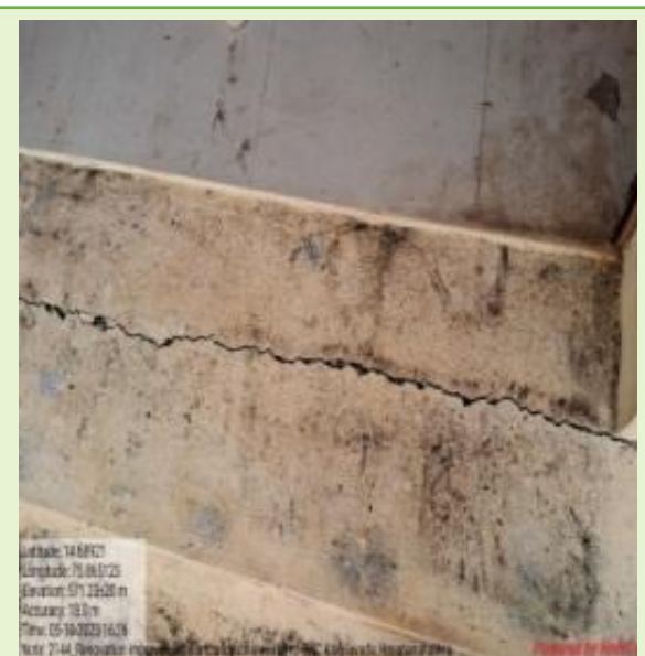
Picture No. 5.12: Cracks in the building repaired through Nirmithi Kendra at PHC Alagilawada, Harappanahalli.
