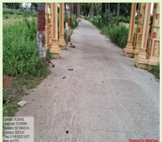
Picture No. 5.11: Non execution of side drainage work in Bhattarahalli Anjaneya Road, Hospete Taluk.
