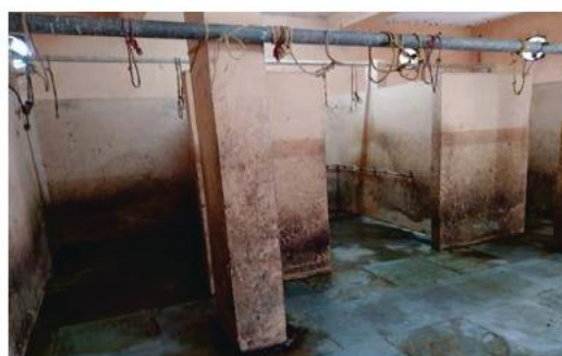
Pictrure 2.2: Walls were not paved with glazed tiles and were not epoxy coated and were unclean at Karaikal
