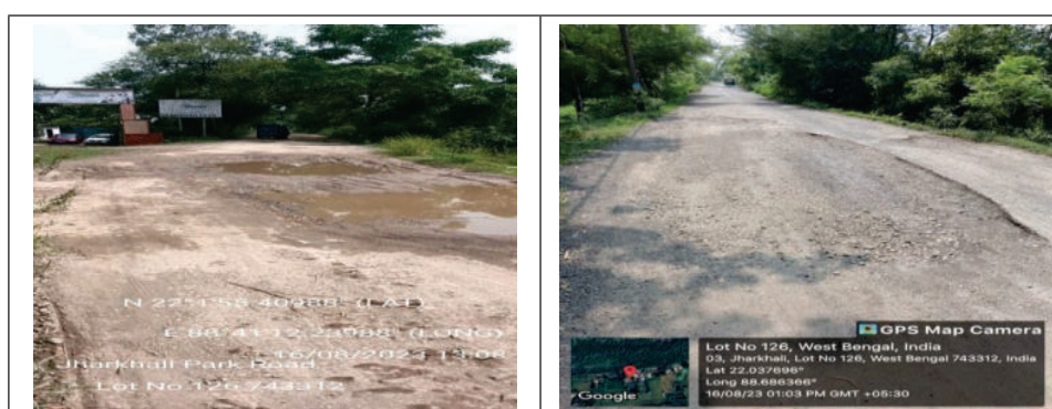
Fig. 3.23: Damaged Road for Jharkhali Eco-Tourism Project, South 24 Prgns.
