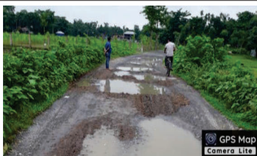
Fig. 4.15: Big size potholes filled with rainwater
