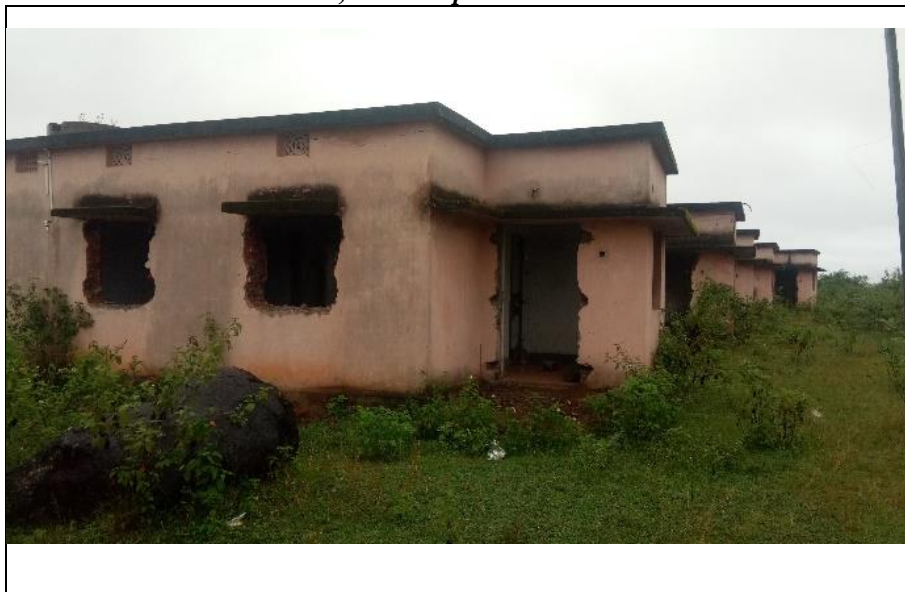
Image 5.1: Dwelling houses, constructed at the Mohanpada village, lying unused, in a dilapidated condition
