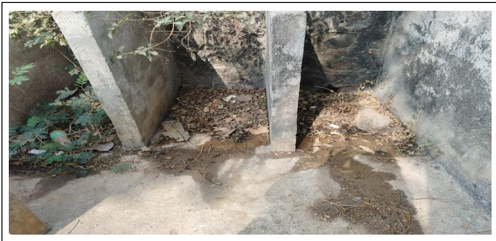
Figure 2 : Unclean and open bathroom at Dnyandeep Boys Hostel, Belora, Mantha, District-Jalna
