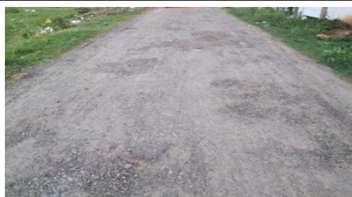
Picture 2.13.1: Damaged surface of NH-16, in front of the Golanthara Police Station to Gadakanallah road (RW Division-II, Ganjam), in the absence of three years' post-construction maintenance
