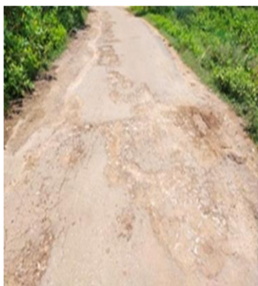
Picture 2.13.3: Crust failure and damaged surface of the PWD Road at P. Jagannathpur to Sunaripalli, in RW-II Ganjam
