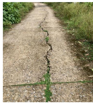
Picture 2.13.5: Cracks visible on the surface of the CC road in Barunasingh to Uttarachaka road, of RW-I Balasore
