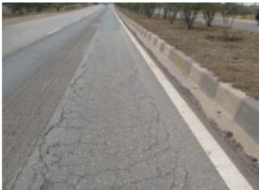
Photo No.14: Crack in BC at RD 73.300
