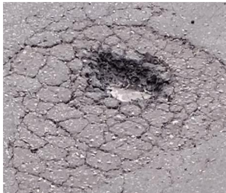
Photo No.12 : Pothole at RD 38.240 km of
