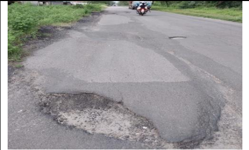
Photo No. 18: Depression at Km 26/125
