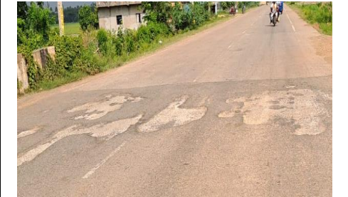
Photo No. 21: Pothole in SDBC on the roof slab of the box culvert
