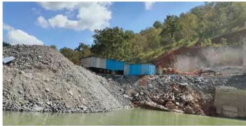
Dumping of excavated muck in Reserve Forest area
