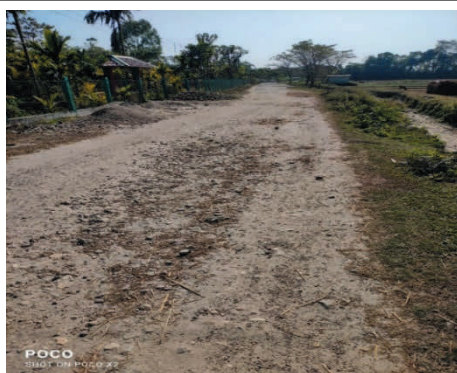
Fig.2.1: Worn out Bituminous surface at 0.5 km of road from Lalpur near Samuktala (20.12.2020)
