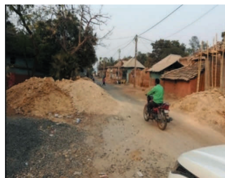
Fig.2.19: Road almost blocked by dumping of construction material at 1.5 km-2.5 km of Seorakuri-Kulkuri Road under Birbhum PW Division (08.03.2021)
