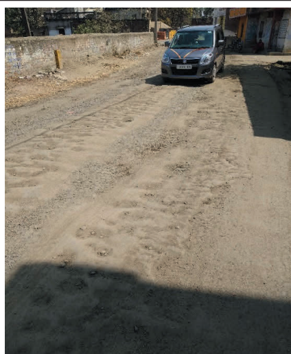
Fig.2.6: Subgrade exposed at various locations of Nalhati Bhabanandapur Road under Birbhum Highway Division-I (27.02.2021)
