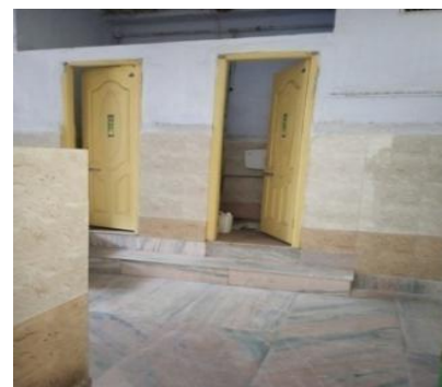
Picture 2.3: Toilets of Hooghly Institute of Technology, Hooghly not disabled friendly
