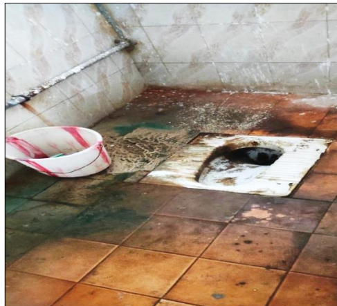
Exhibit 3.7: Unclean toilet at Urban PHC, Vettavalam
