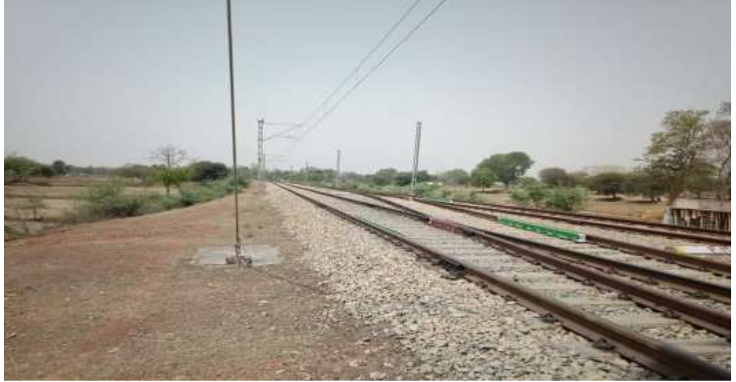
Incomplete wire stringing work
