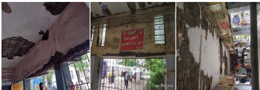
Hospital building is about to collapse in DH-Jehanabad
