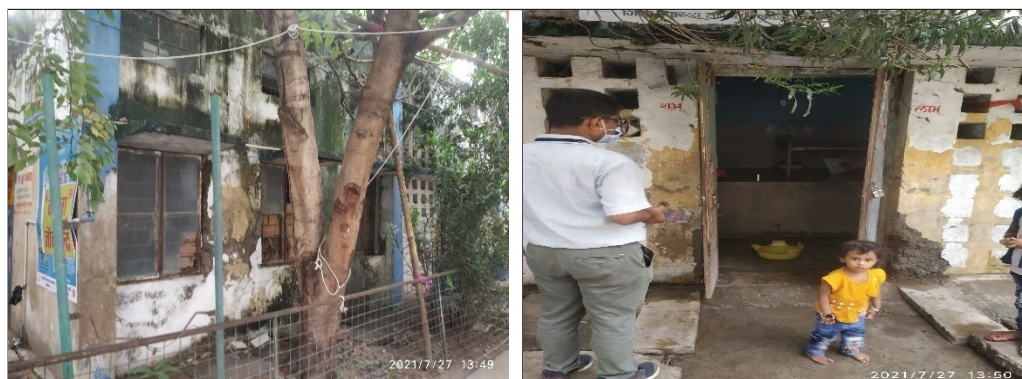
Kitchen at DH-Jehanabad in a condemned building
