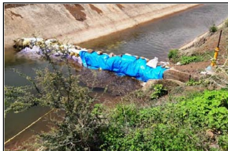
Artificial obstruction in LBC for feeding direct minor-13 (status as on July 2017)
