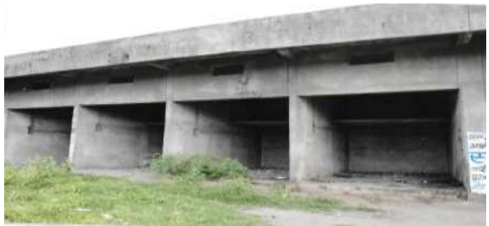
Photographs showing incomplete and idle shops at Kumhari
