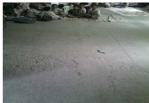
Picture 8 : Poor flooring at Sathuvachari West Primary School
