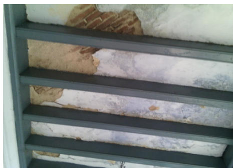
Picture 7: Damaged roof of Corporation Middle School, Kalasapalayam
