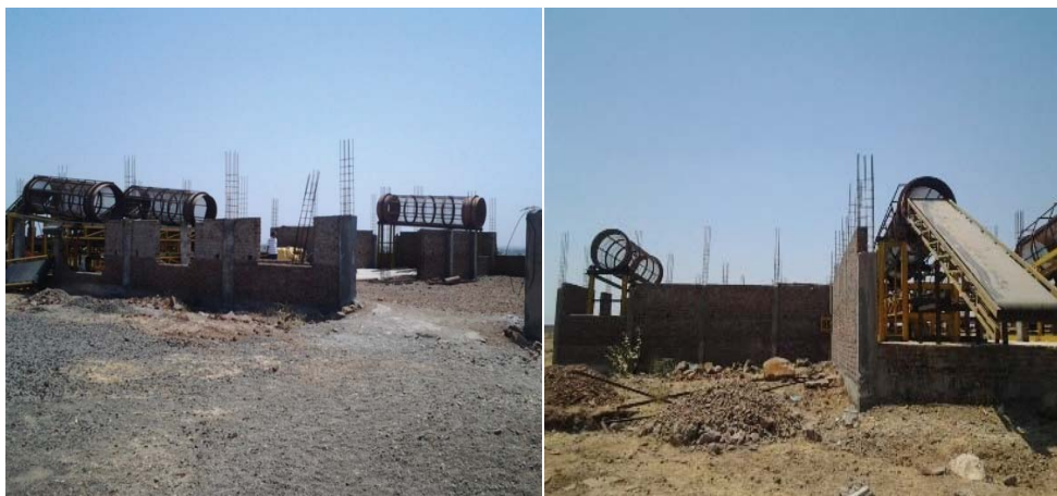
Waste processing facility in Jalna, Maharashtra
