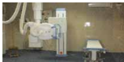
Picture 3.8: Digital X-ray not commissioned at MCH, Vellore.
