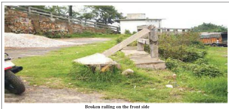
Broken railing on the front side
