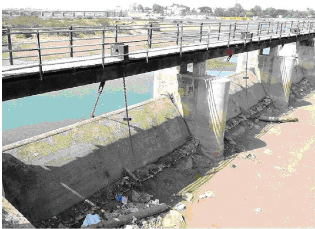
(Photograph showing non-functioning of Gates due to trash/bushes getting stuck in the axle)
