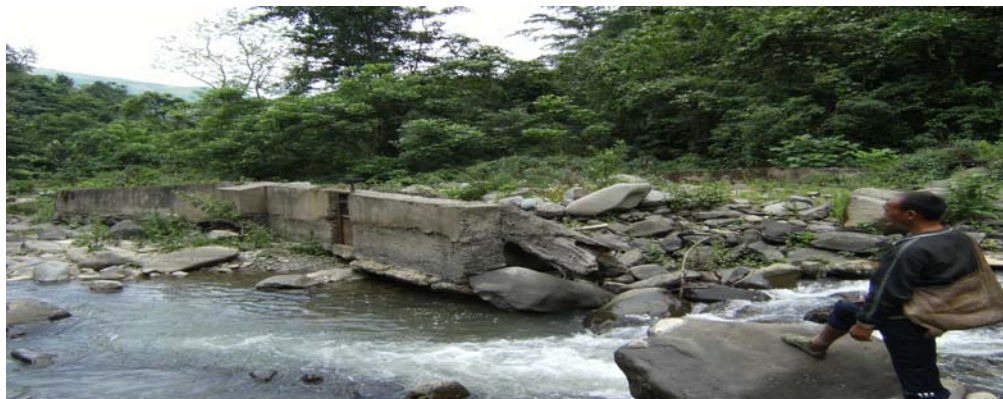
Photographs shows the present position of the Lamong MI project under RIDF.
