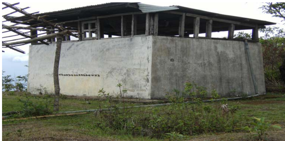
Photograph showing the present status of Main reservoir cum distributor of Thizuru project
