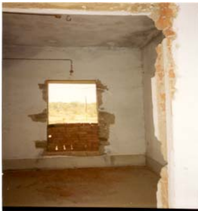
Stolen door frame and missing window frames
