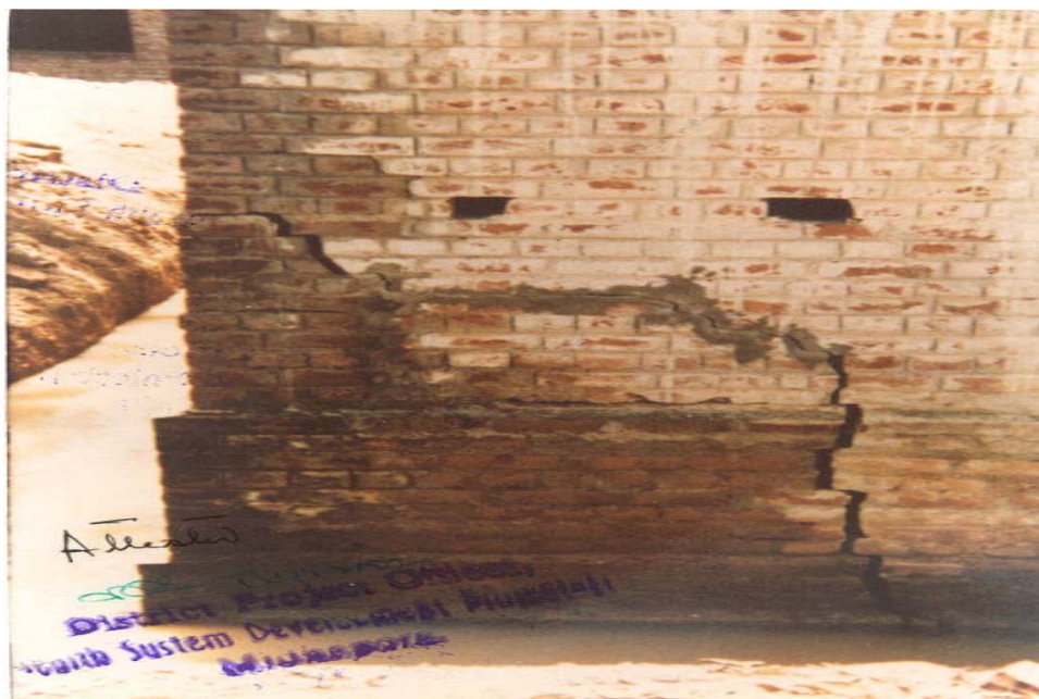
Cracked foundation and plinth of Binpur Rural hospital due to water logging
