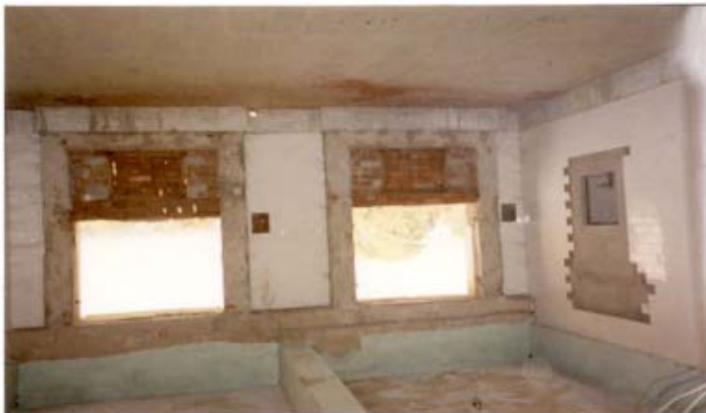
Missing windows, empty ward and damaged roof plaster
