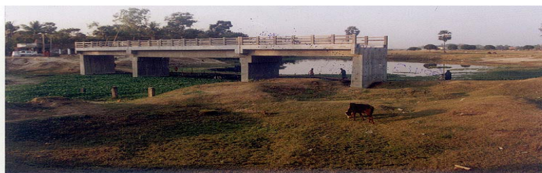
Incomplete construction of Subarnamgiri bridge and approach road at Bhagawangola block in Murshidabad remaining abandoned since March 2003
