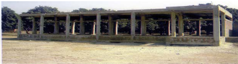
Incomplete construction of Aurangabad High Madrasa at Suti-II block of Murshidabad remaining suspended since January 2005
