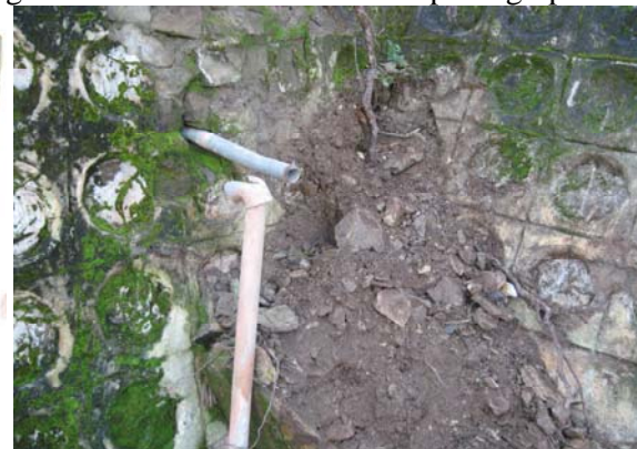
Picture: 3.1.8 Broken Intake Pipeline
