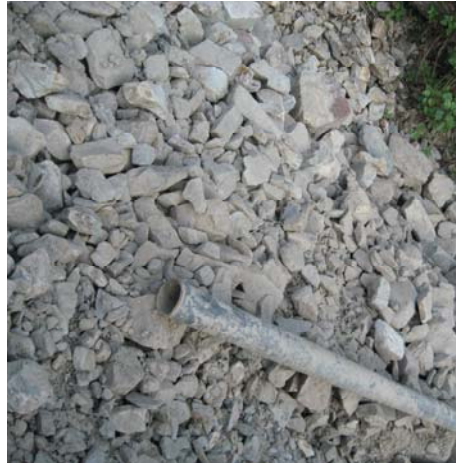
Picture: 3.1.10 Broken Intake Pipeline
