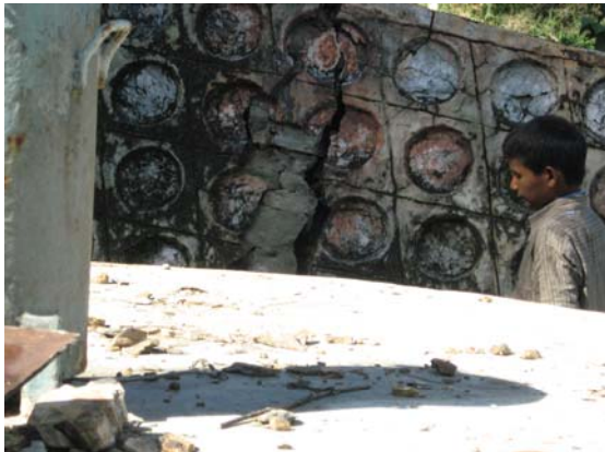
Picture: 3.1.6 Cracked Pushta
