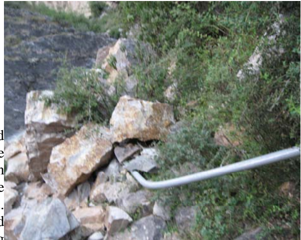
Picture: 3.1.11 Hanging line prone to falling boulders
