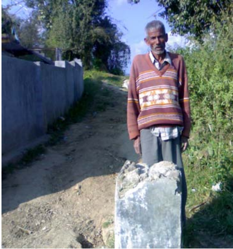
Pic: 3.1.13 Broken Stand Post without pipe
