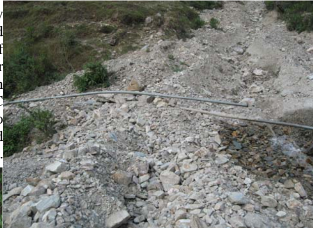
Picture: 3.1.9 Broken Intake Pipeline
