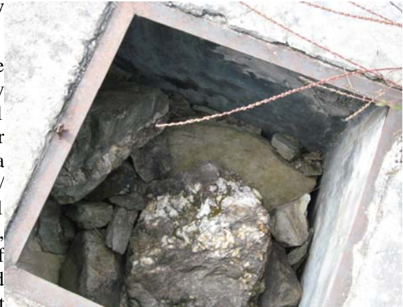
Picture: 3.1.2 Water Intake Tank
