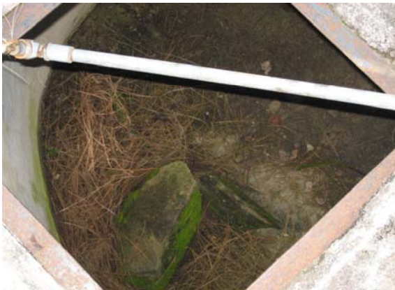
Picture: 3.1.3 Supply Tank
