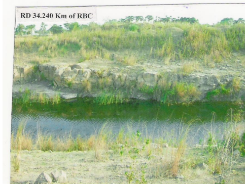
(Failure of slope and slippage of embankments at RD 31.55 to 34.24 km of RBC)
