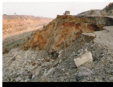
(Bank sliding at RD 34.10 to 34.20 km of LBC)
