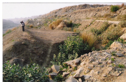
(Bank sliding at RD 33.57 to 33.67km)
