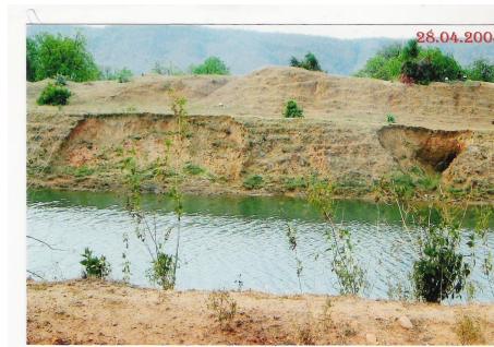
(Damaged canal embankment at RD 8.00 km to 8.04 km due to absence of CC lining)
