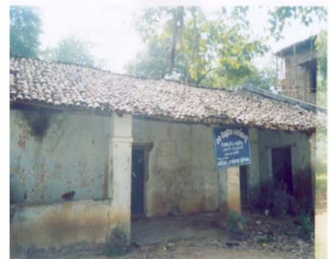
Dilapidated office building of the Gudighat watershed in Muribahal Block (Bolangir district)
