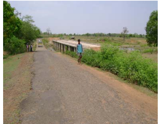
Bridge over river Bankal at 1 st km on Banki-Badamitalia road completed without construction of approach road
