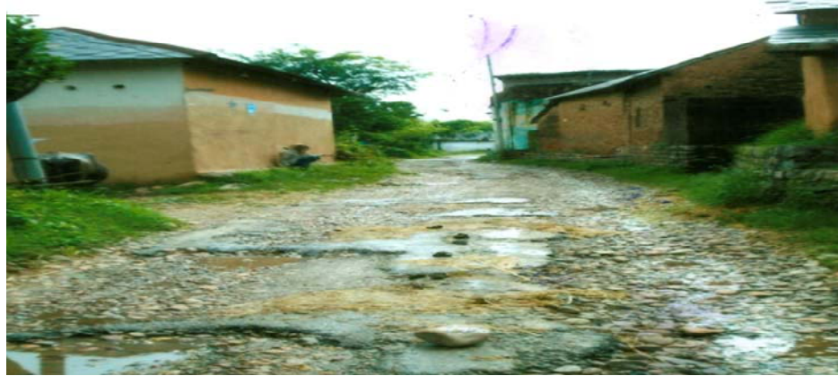
Damaged Bhogarwan Samlet road due to non-construction of side drains
