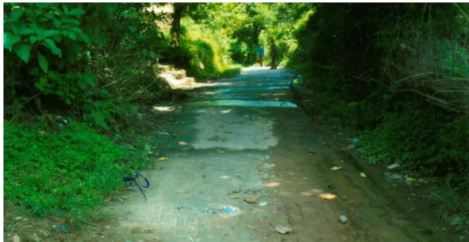
Damaged Dadwalah via Rehan Bazar to Sakari road due to non-construction of side drains
