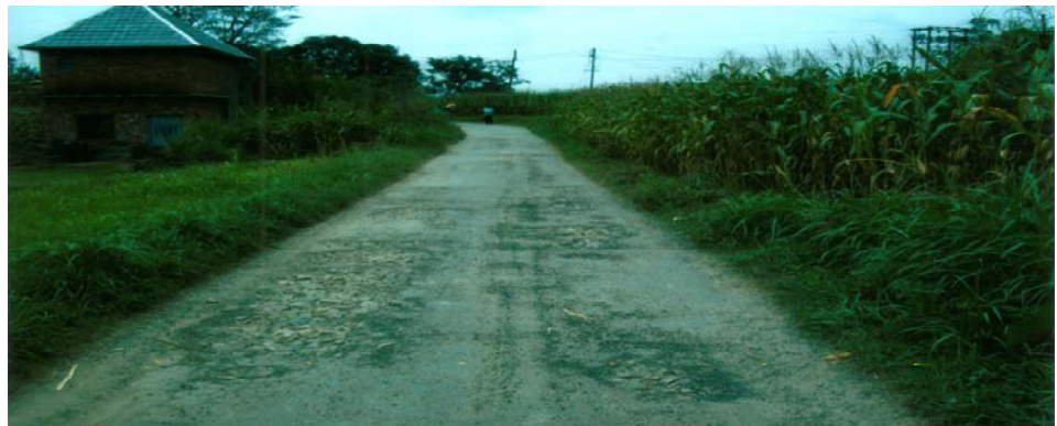
Damaged crust of Rohal khad to Ghandalwin road via Lahri Sarail (RD 5/765)
