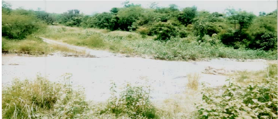
Unutilised Gopipur Chamukha road due to non-planning of a bridge over Balahar khad
