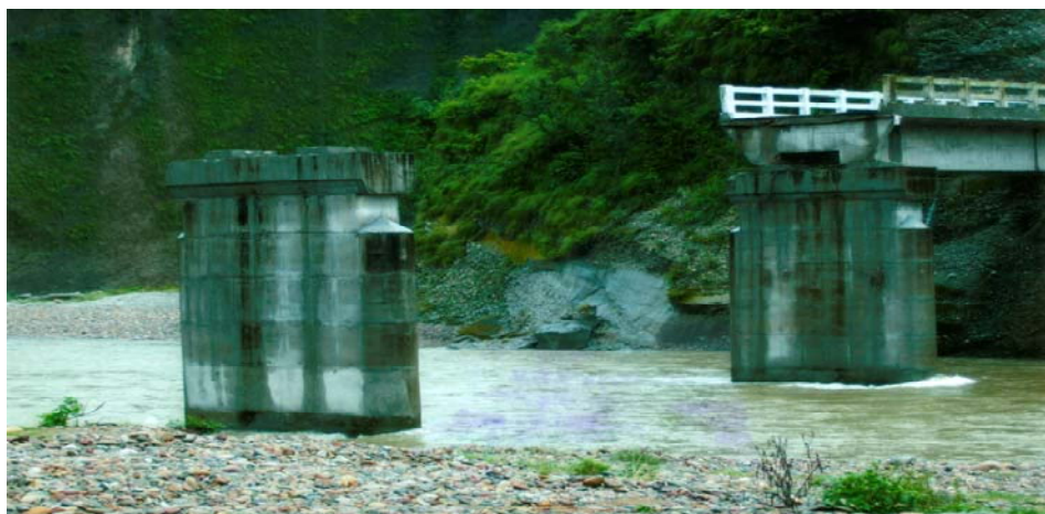
Washed away Bridge over Seer khad on Bara-Da-Ghat Kuthera road via Bhapral-Talwara
