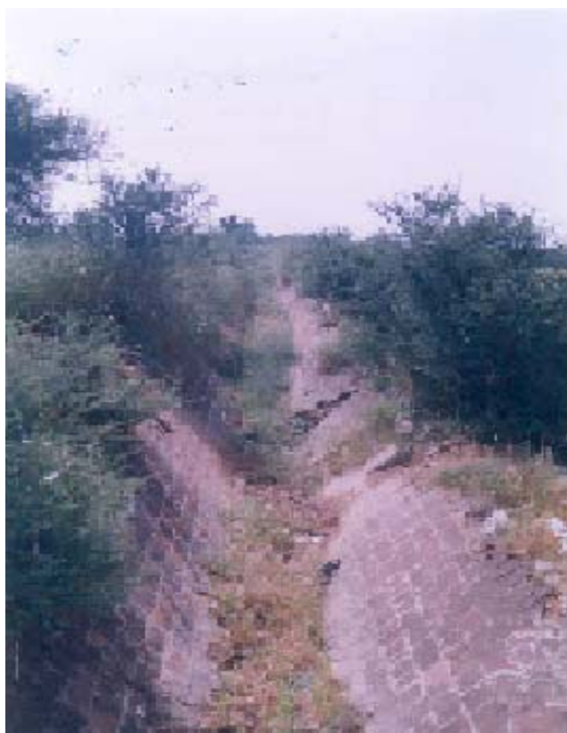
Non-functional Saleempur Minor RD 4,500 (Sr. No. 4 of Appendix XV )
