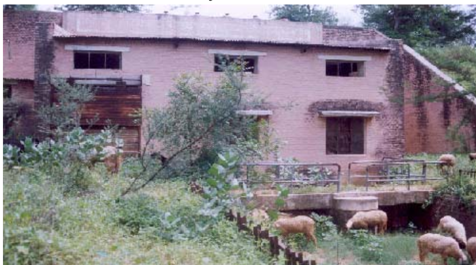
Non-working pump house No. 7 at Dewana Distributary km 29.313
