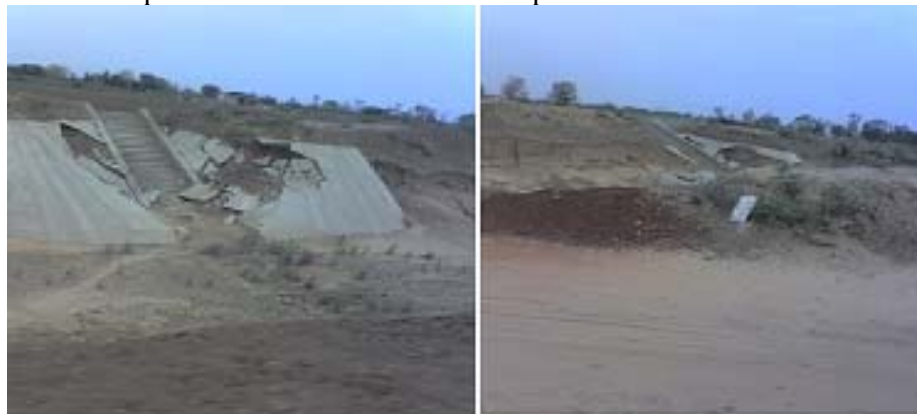
Picture 3: Structures in SSSC damaged during monsoon
