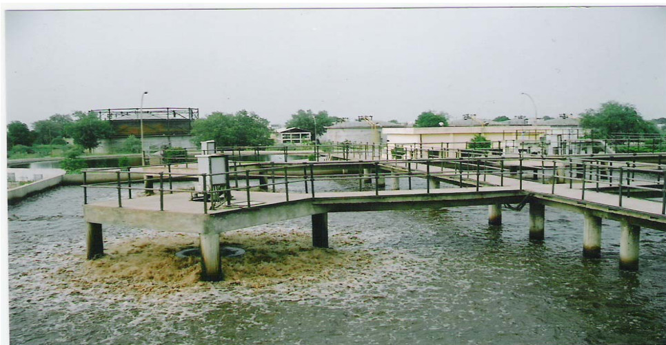
Figure-10: A view of sludge treatment at a sewage treatment plant
