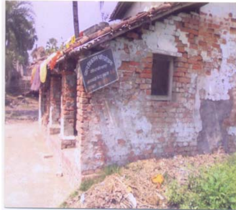
Unsafe and dilapidated Anganwadi Centre at Dhuiya Tola under Cheria Bariyarpur Project, Begusarai
