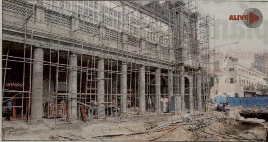
RUNNING AROUND IN CIRCLES: Restoration of the façade in run-up to the 2010 Games was done only in outer and inner circle at a cost of Rs 40.02 crore, while middle circle was not covered, the CAG report said
