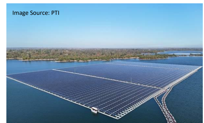
Image: Omkareshwar Floating Solar Park, Khandwa Madhya Pradesh
