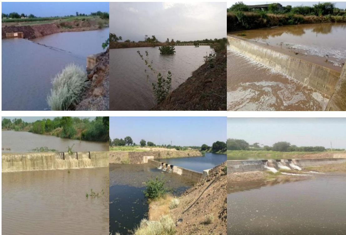
Figure 17 Series of Cement Nala Bund (Kolhapur padhatiche Bandhare) at Jawalarjun under the SAGY 15 .
