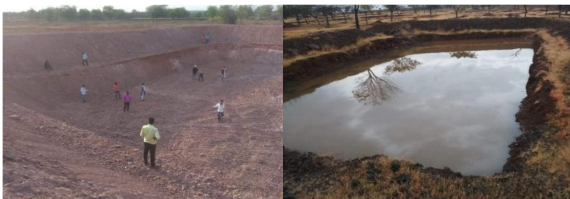
Figure 14 4 Farm Pond (Shet Tale) in Jawalarjun Village, (Water level). Before and after of structure 5
