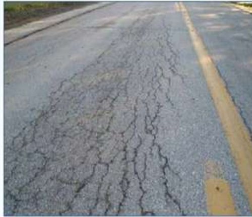
Figure 1.1: Crack of pavement due to Fatigue strain
