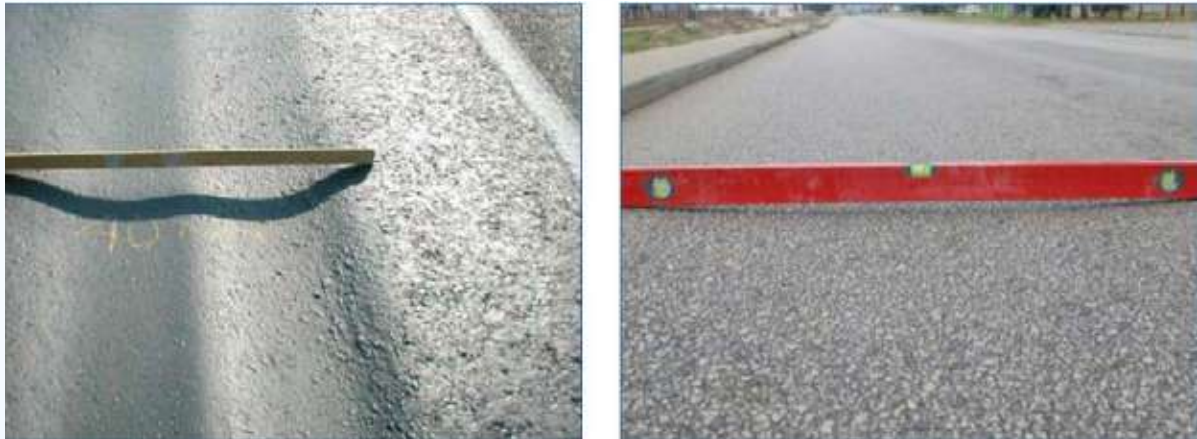
Figure 1.2: Surface depression due to rutting strain
