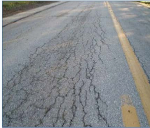
Figure 1.1: Crack of pavement due to Fatigue strain
