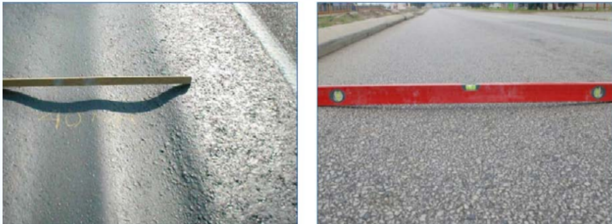
Figure 1.2: Surface depression due to rutting strain
