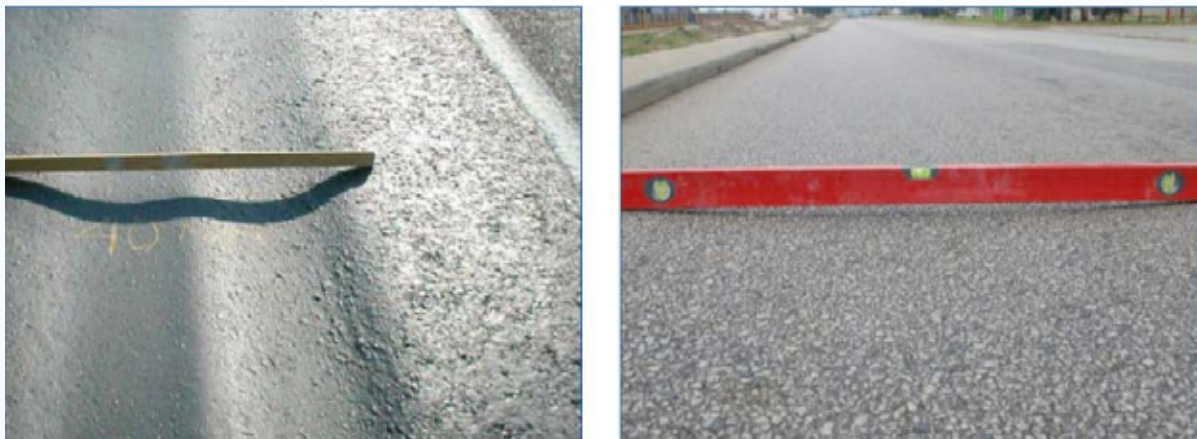
Figure 1.2: Surface depression due to rutting strain
