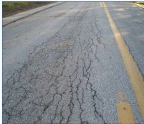
Figure 1.1: Crack of pavement due to Fatigue strain
