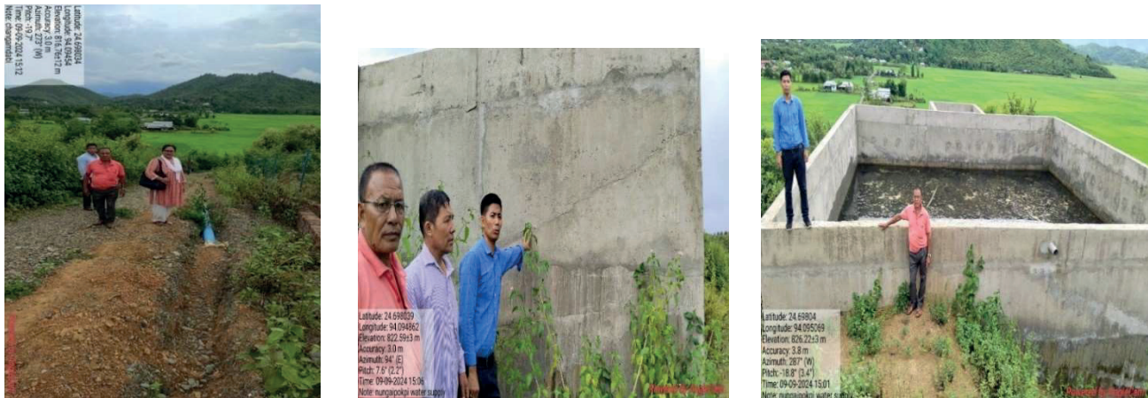
Laying of pipe in middle of road Development of crack in reservoir wall No compound wall
