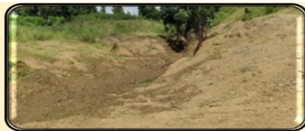
Pic 6.4: Picture taken during JPV, which indicates that the Amrut Sarovar lacks a proper water retention structure, like construction of rock toe, puddle filling, etc. required as per Technical Sanction, making the construction expenditure ineffective. The pond was found dry even in the rainy season, raising doubt about authenticity of the work executed and its completion certificate.
