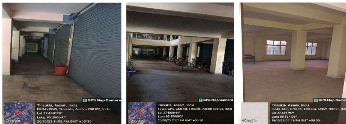
Present status of unused floors of the Commercial-cum-Office Complex under Tinsukia MB
