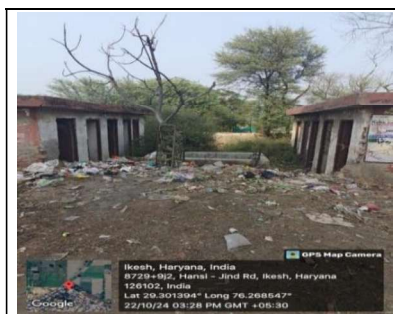
Image showing dilapidated condition of public toilets in Village Ikkas, Block Jind, District-Jind
