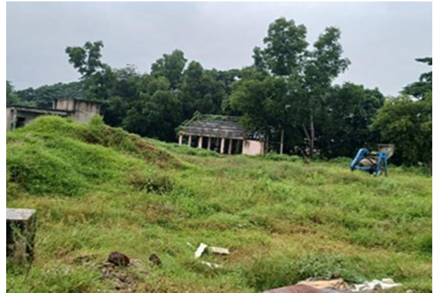
Picture 3.4.3: Uneven and unmaintained surface of Mini stadium at Pipili (Date: 22 August 2024)
