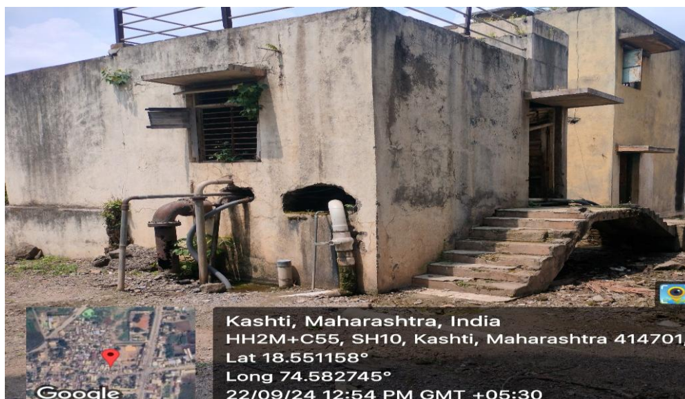
Photograph 2: Unused WTP in Kashti village of Shrigonda block
